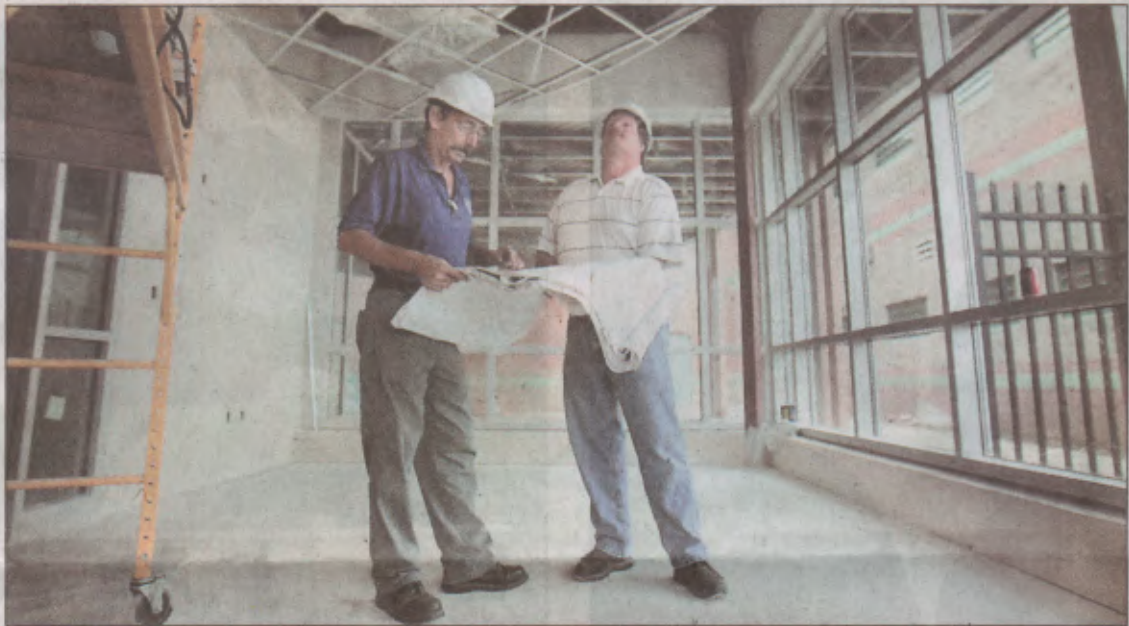
Tom Dadisman (left) and Mike Wassenich from St. Vincent Hotel look over blueprints in the Gettysburg Gateway for Men shelter, which is set to open Oct. 16. Staff photo by Jim Witmer
